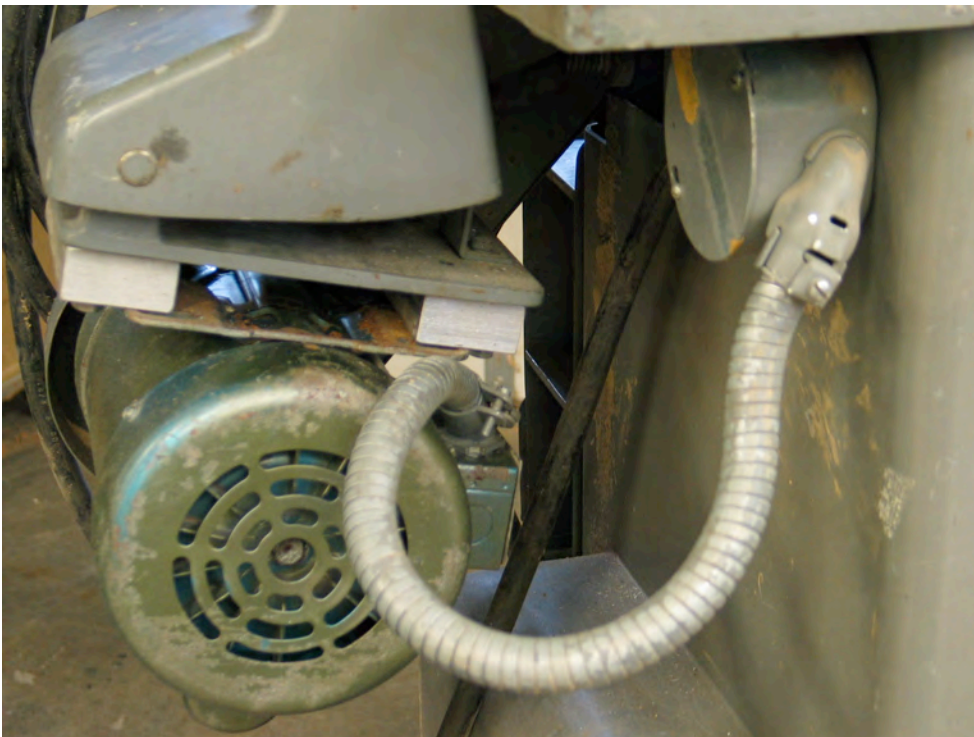
Figure 49 The 56 frame, 3450 rpm motor installed
