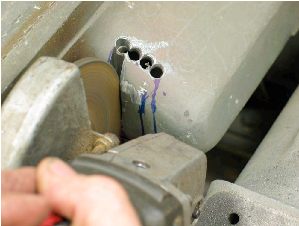
Figure 267 A 4-1/2" angle grinder does quick of cutting a slot up to the holes.
