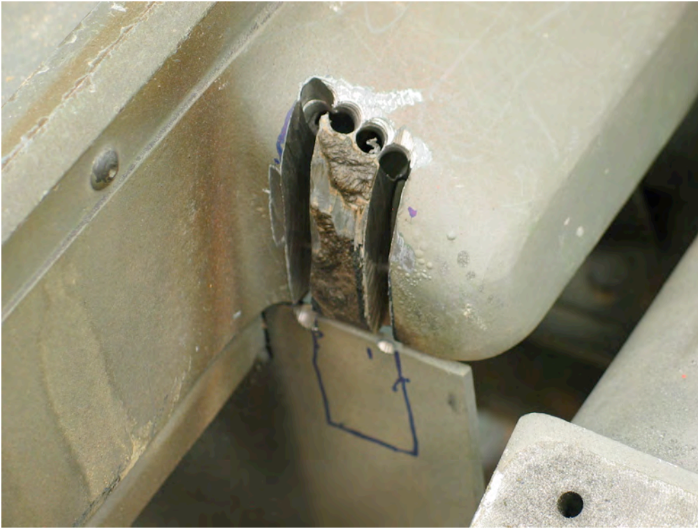
Figure 278 Slot s are not cut and the opening is ready for removal.
